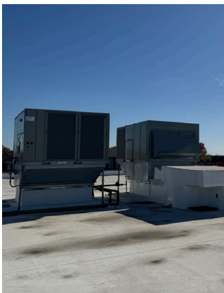
New rooftop HVAC equipment at the Paterson facility improves energy efficiency, reliability, and comfort for daily programs and activities.
