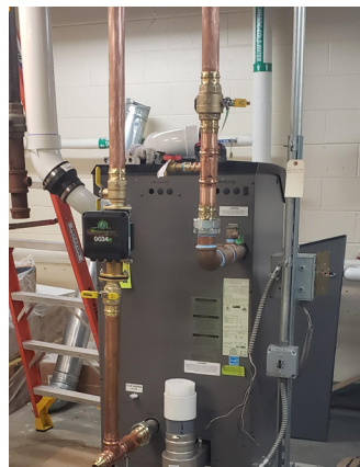
The new high-efficiency boiler helps improve system reliability while reducing energy use and operating costs.
