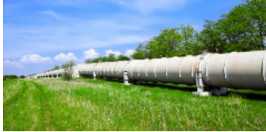
Interstate Natural Gas Transmission Line
