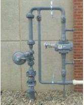
Customer Gas Meter
