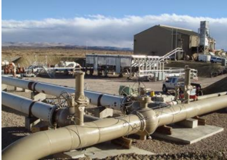
Natural Gas Metering & Regulating Station
